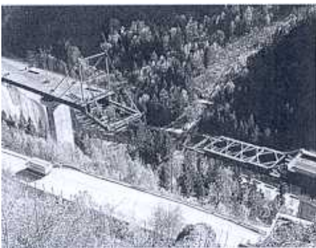
Fig. 5.5.15: Connection of the bridge parts, built in two different yards (Aosta and Mont Blanc sides)
